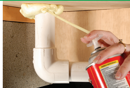
SAVE ENERGY: Expandable foam acts as an insulator, sealing holes around pipes and fixtures.
