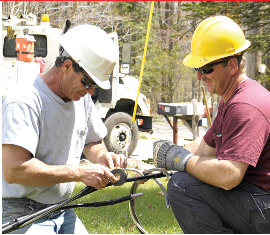
ABOVE: Martinsburg district Crew Chief Greg Dilling, left, and Journeyman Lineman Rob Shook splice secondary underground wire for a service upgrade along Coppock Road.
