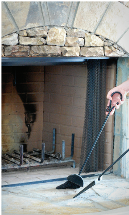
COZY YET COSTLY: Fires are a low-efficiency, high-maintenance source of heat requiring constant tending and ash removal.
