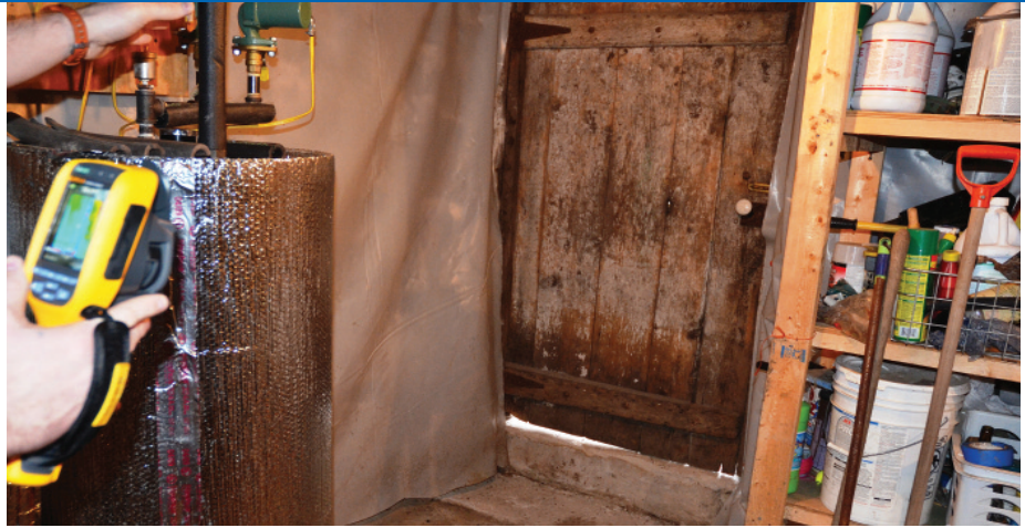
CHECK EVERYTHING: The insulation wrap on the water heater is a good energy-saving start, but the old cellar door is hemorrhaging heat. Where you see daylight, you're seeing heating/cooling loss.
