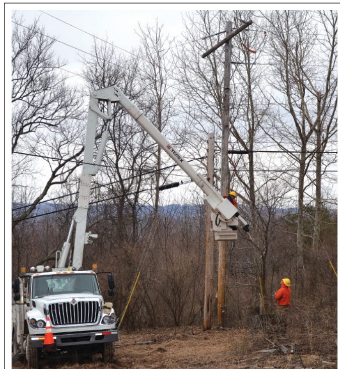
INVESTMENT: Valley REC line crews in April set new poles and string new wire along School House Hollow Road in Henderson Township, Huntingdon County. The upgrade is part of a 2013 work plan project that will continue into the fall. Crews completed the initial work with minimal interruption of service to members. (Photo by Doug Roles)
