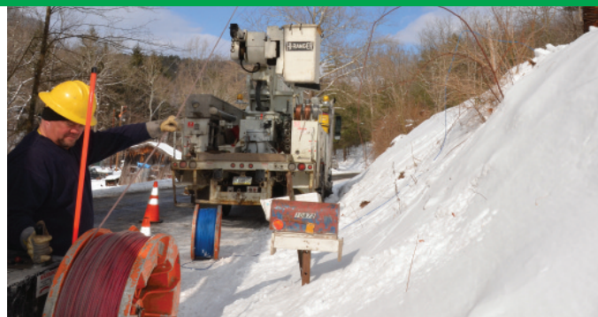
HARD AT WORK: Valley REC equipment operator Rich Sunderland feeds high-tension rope from a spool in February in Henderson Township, Huntingdon County. The rope is used to pull new wire into place. The work by Valley crews to string new line is part of the 2014-17 work plan.
