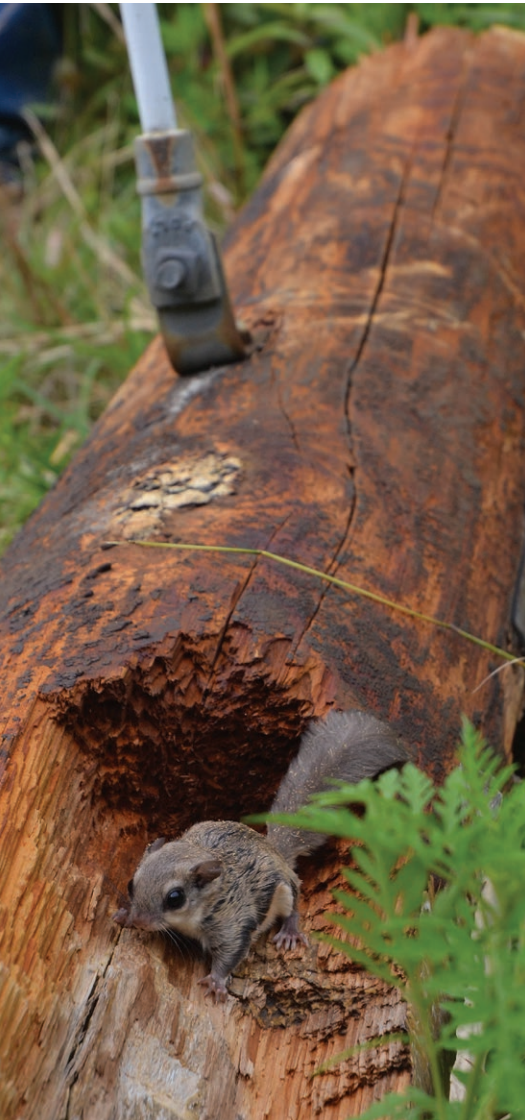
NO PLACE LIKE HOME: A flying squirrel figures out its next move after crews lower the top of a damaged pole to the ground. This pole was damaged so badly by woodpeckers that it had to be replaced.
