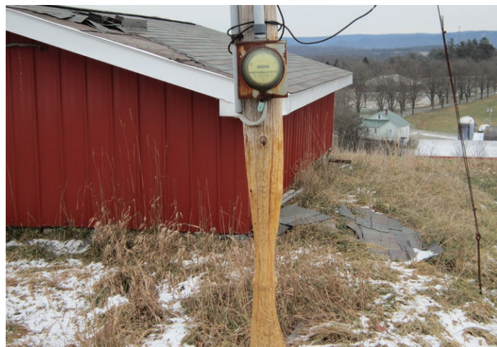
RUBBED DOWN: Something’s not quite right here! It looks like the work of a beaver, but actually it was the resident deer at Pine Tree Trophy Whitetails, LLC in Fulton County that rubbed this pole to the core. A pole this badly damaged poses a serious hazard.
