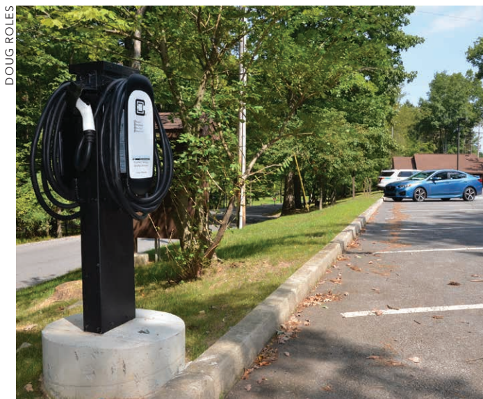
POWER UP: An electric vehicle charging station stands ready at Cowans Gap State Park.
